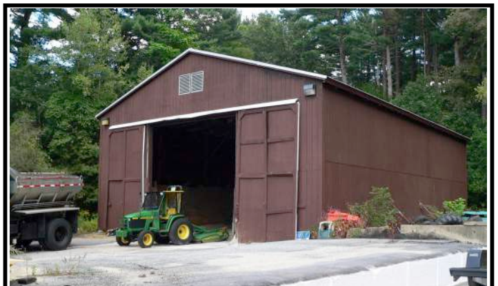
Fig. 27: Road salt shed, built in 1988, replaced a dilapidated structure that had been used for many years.. Photo, J. Hauck, 2014.
