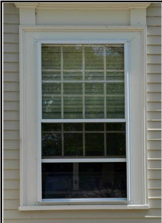
Fig. 31: Distinct change to town hall exterior frame with the installation, in 1993, of aluminum storm and screen windows. Photo, J. Hauck, 2014.
