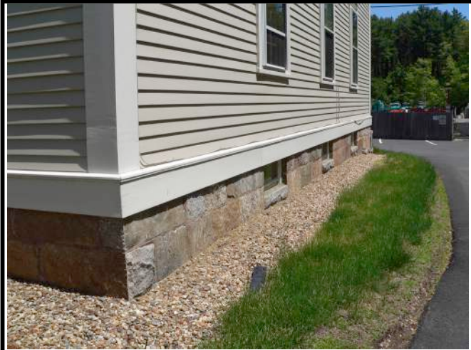
Fig. 20: Around the entire foundation, below each of the first floor windows, there were fixed, basement windows, with stone sills, Photo, J. Hauck, 2014
