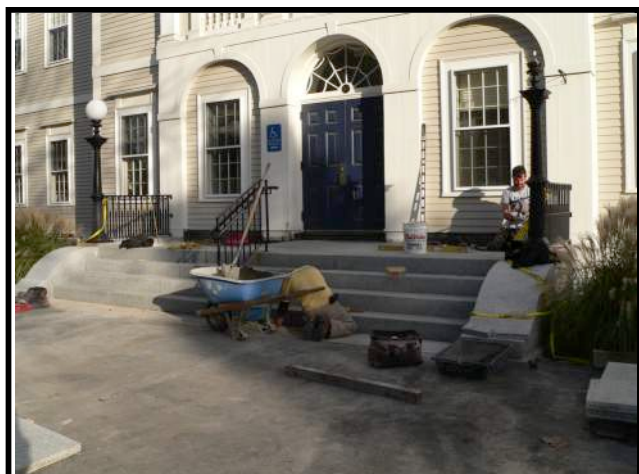
Fig. 33: Granite front steps repaired in late 2014 to eliminate uneven surfaces. Photo, J. Hauck, 2014.
