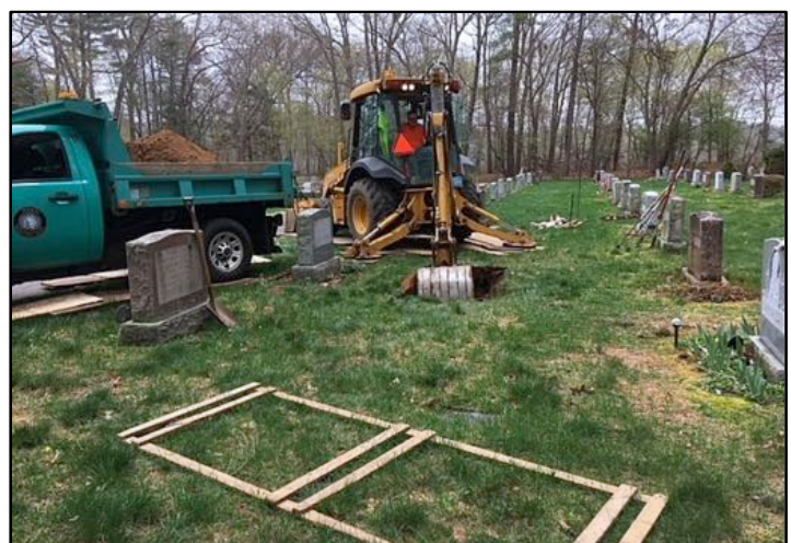
Backhoe replaced grave diggers. Wood form is used to check depth and width of grave. Photo, J. Hauck, 2018.
