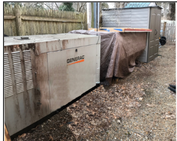
Equipment storage area, beside addition, has equipment shed and a backup electric generator.
